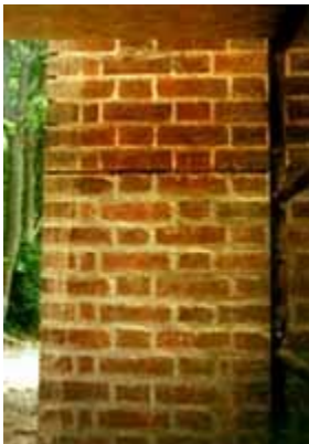
A mechanical grinder improperly used to cut out the horizontal joint and incompatible repointing have seriously damaged the 19th
