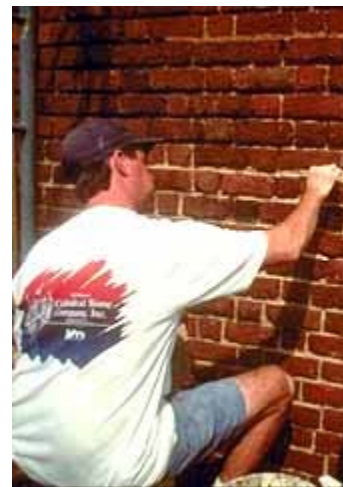
This early 19th century building is being repointed with lime mortar. Photo: John P. Speweik.
